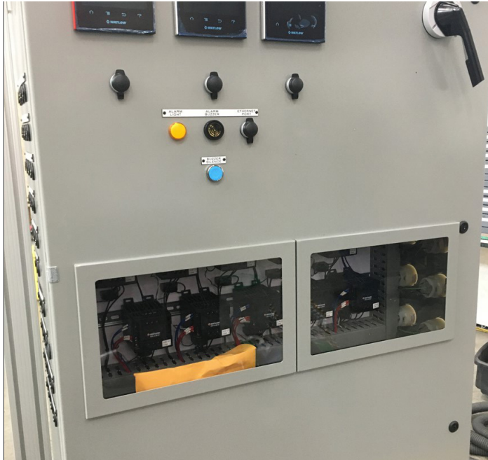
Front of Control Panel
